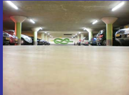
Premium Power LED in parking garage Houtplein, municipality of Haarlem, The Netherlands
