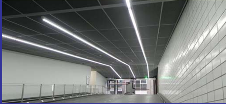
Premium Power LED Lines in parking garage The Bank, park King Amsterdam The Netherlands
