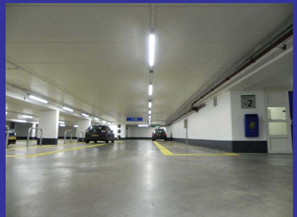
Premium Power LED in parking garage Bios, Interparking, Groningen, The Netherlands
