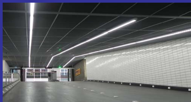
Premium Power LED Lines in parking garage The Bank, Park King Amsterdam, The Netherlands (covering long distances)
