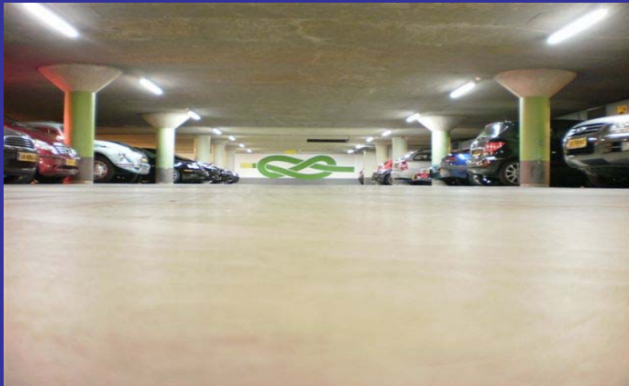
Premium power LED lighting in parking garage Houtplein, municipality of Haarlem, The Netherlands
