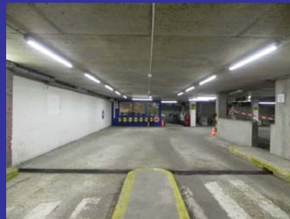
Premium Power LEDs in parking garage Oosterpoort, municipality of Groningen, The Netherlands
